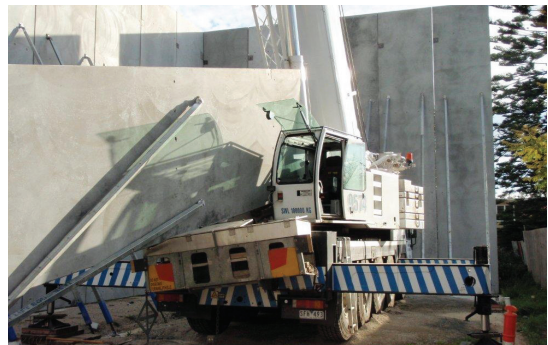
A rigger suffered a serious hand injury and a crane operator narrowly avoided death when a lifting insert fell out of this panel on a Charnley Vale site in Brunswick on 1 August.
